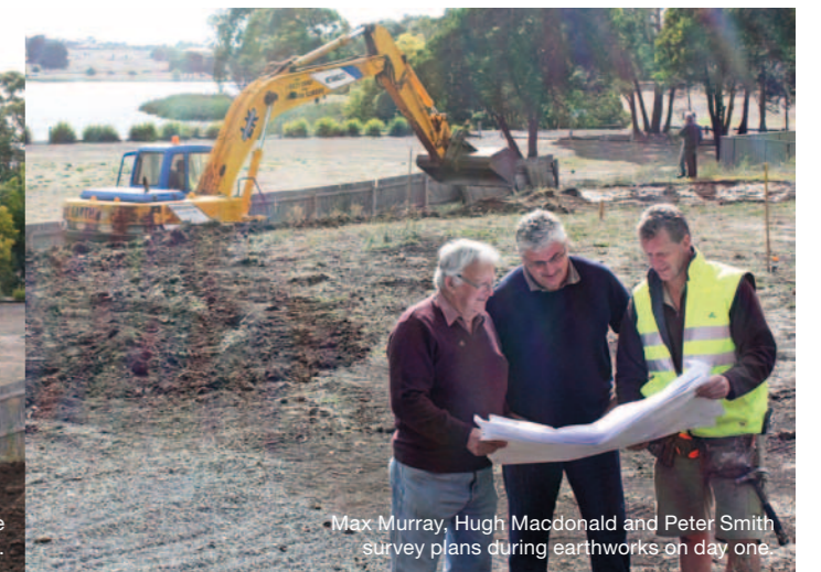
LK Earthmovers turn earth for the first time on the Watermark Charity House site.
